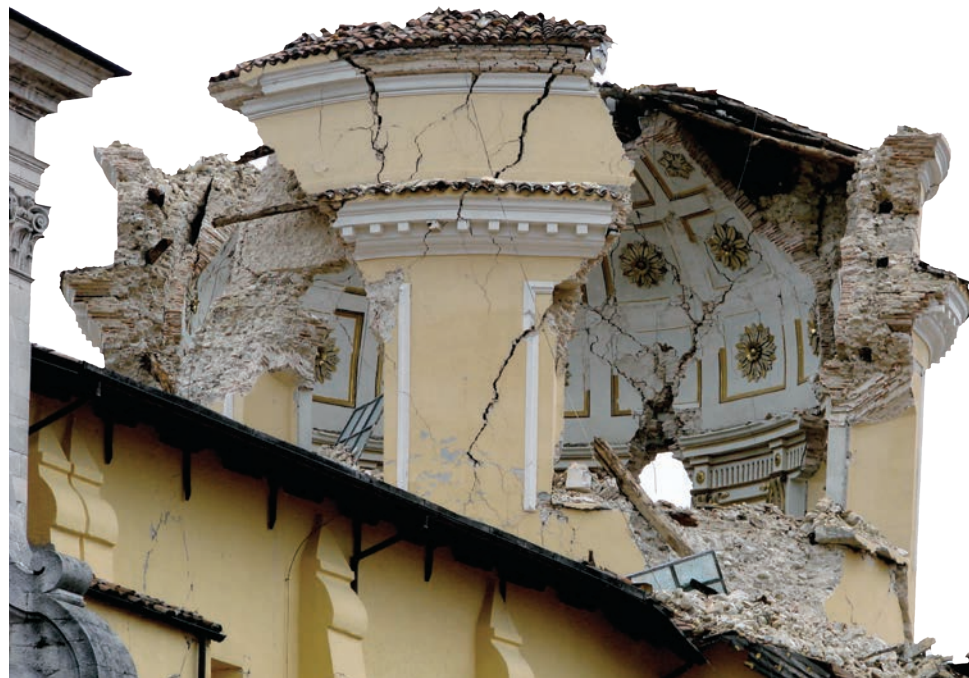
Chiesa delle Anime Sante. Damage to the dome of the Church of the Holy Spirit in L'Aquila following the 2009 earthquake. PHOTO: UCL MATHEMATICAL AND PHYSICAL SCIENCES - LICENSED UNDER CC BY 2.0
