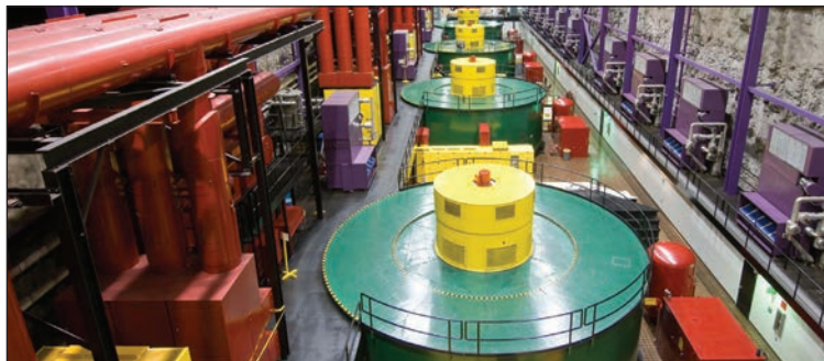
The Raccoon mountain powerhouse.
